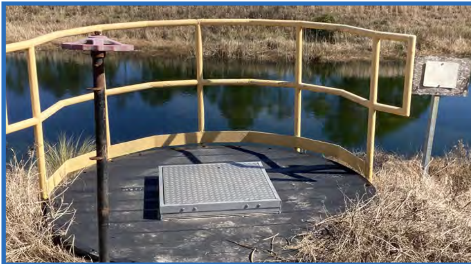
Leachate Collection and Leak Detection System Manhole for Increment 1
