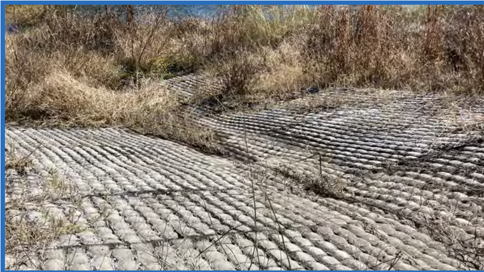
Fabriform-Lined Flume into Stormwater Pond B, Looking Southeast
