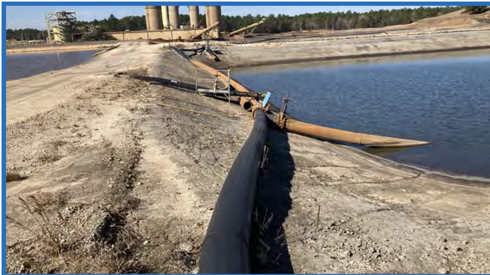
Discharge of Pipeline in Previous Photo into Pond 9, Looking West Along Dike Between Ponds 3 and 9
