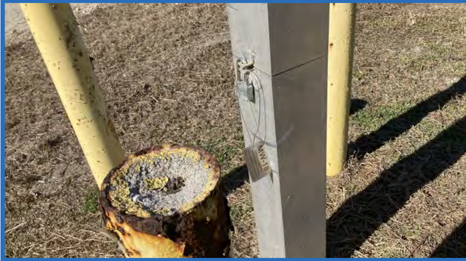
Monitor Well MW-18 and Protective Bollards
