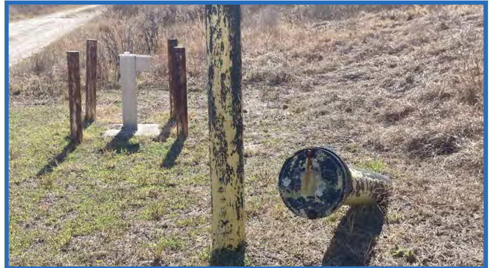
Monitor Well MW-22 and Leachate Collection System Cleanout East of Perimeter Road, Looking South
