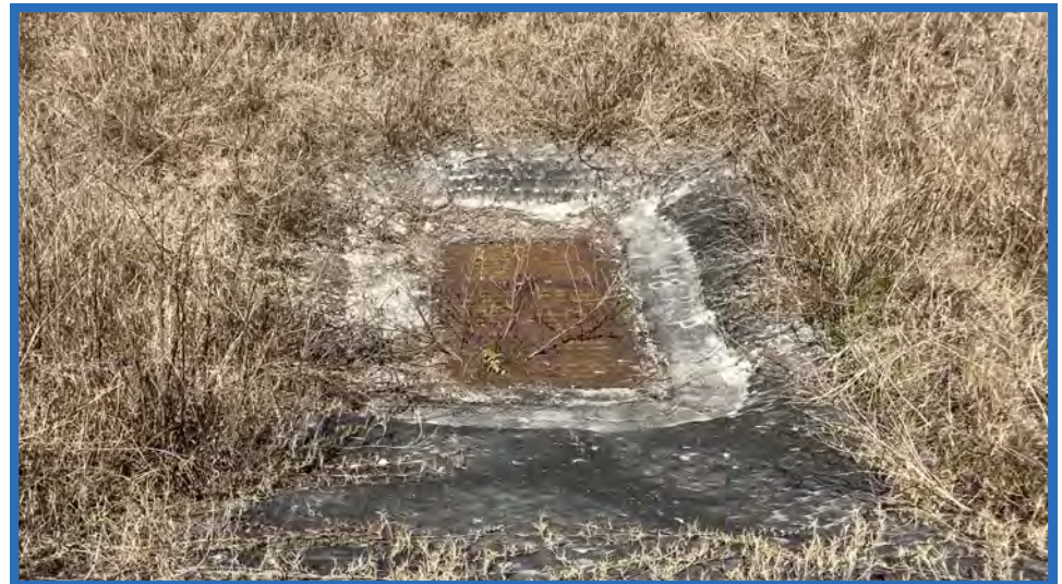
Stormwater Inlet in Southeastern Corner of Increment 1
