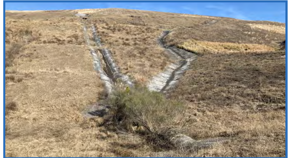
North End of Western Containment Dike for Stage IIB and Fabriform-Lined Flumes, Looking North
