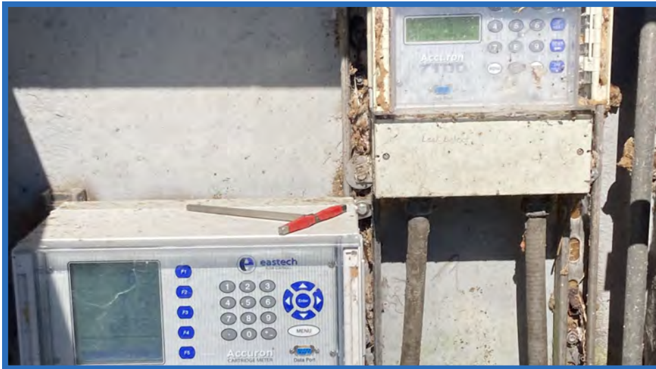
Leachate Collection (Left) and Leak Detection (Right) Flow Meter Control Panels for Increment 1
