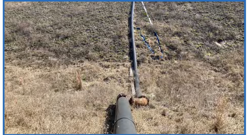
Pipeline from Auxiliary Pumps for Low Point of Stage IIB to Pond 9, Looking East
