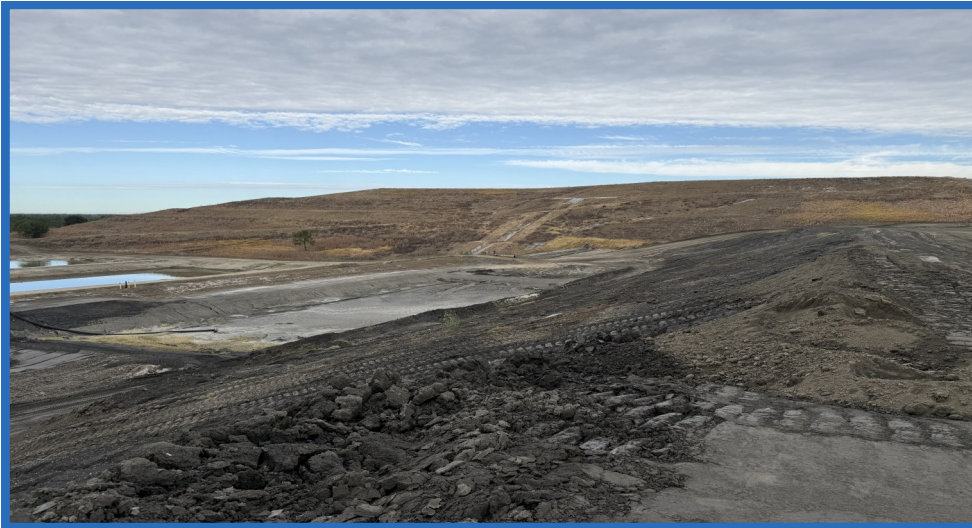
Pozzocrete Dike and Low Area on West Side of Increment 1 (Looking Northwest)
