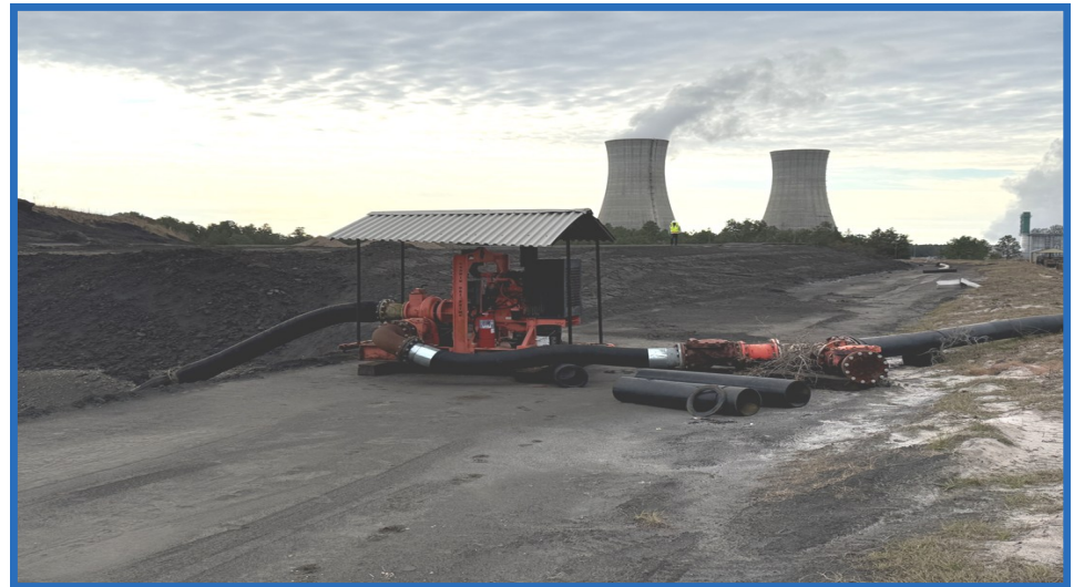
Auxiliary Pump on West Side of Increment 1 (Looking Southeast)
